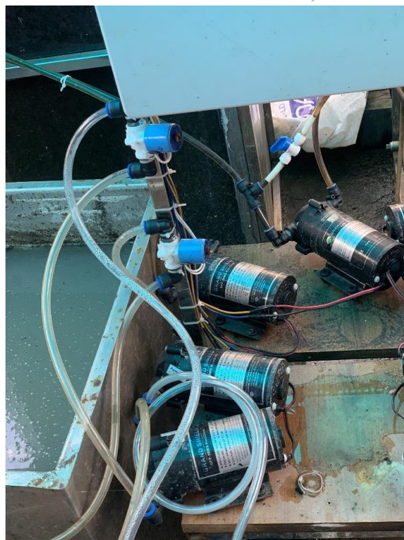
Figure 27: Pump and Valve attached on the stander
