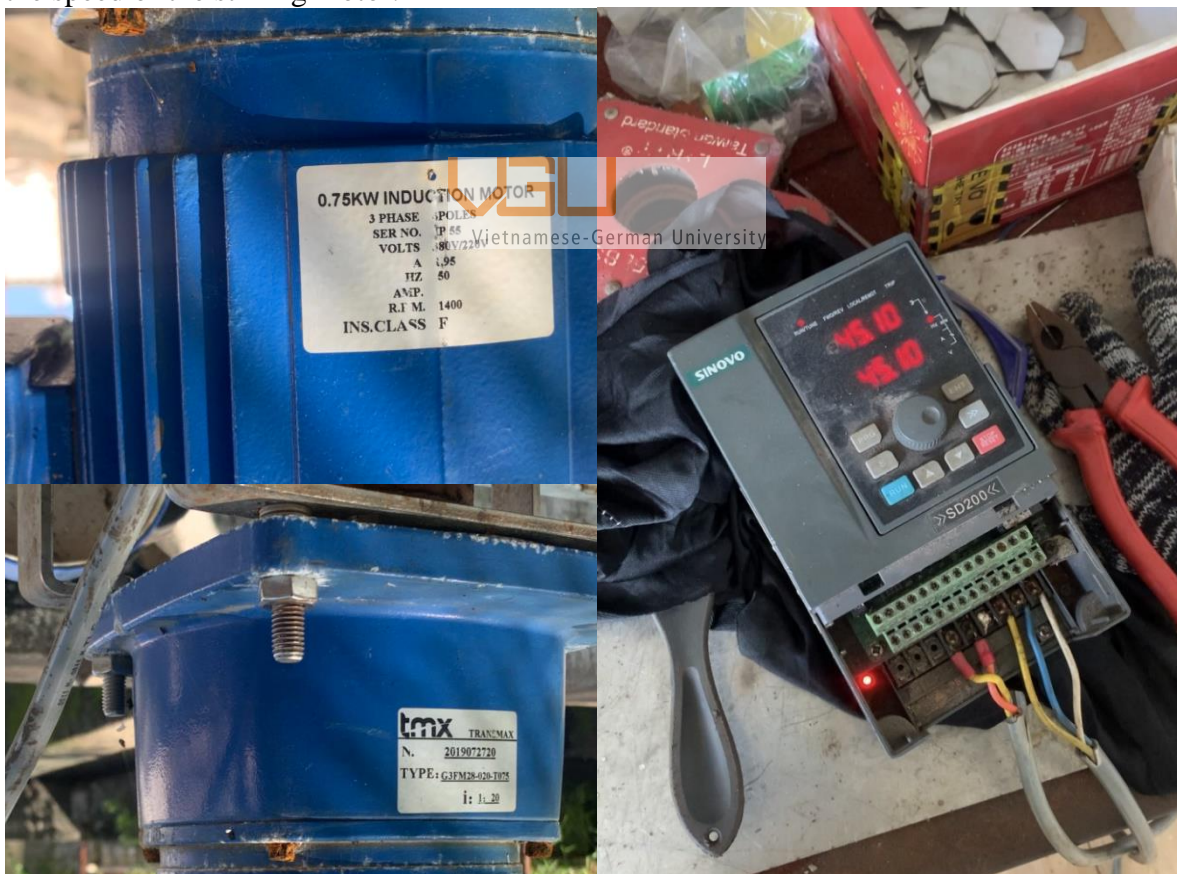
Figure 17 Motor with gear box and inverter for stirring design
