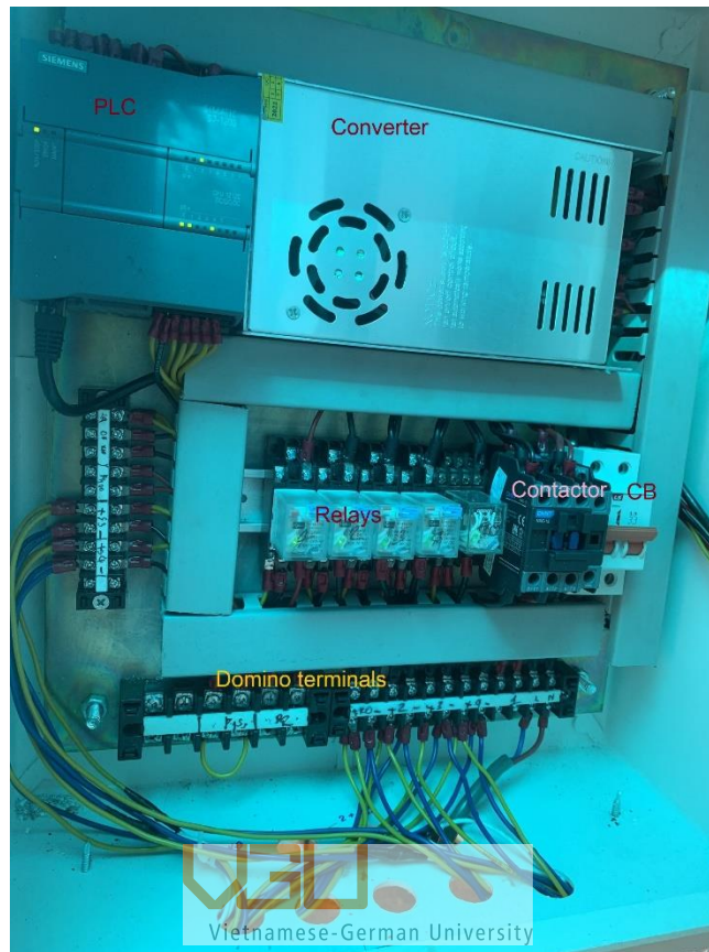
Figure 30: Electrical cabinet after finish
