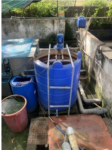
Figure 20: the finish stirrer and pretreatment tank
