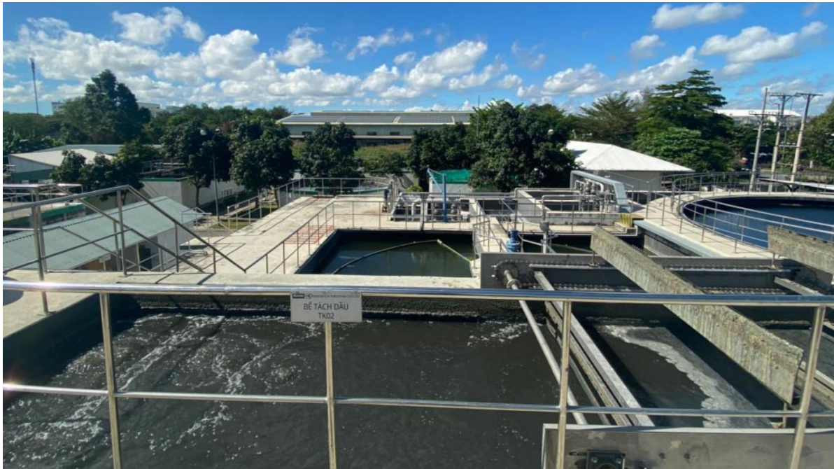
Figure 2: Oil and grease separating tank
