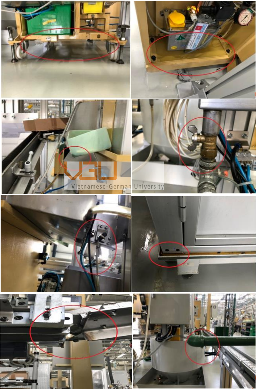
Figure 2. Oil leaking spots
