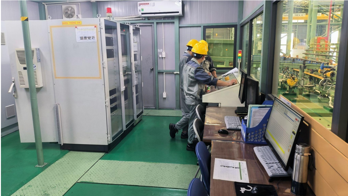
Figure 8: NDT Control Room
